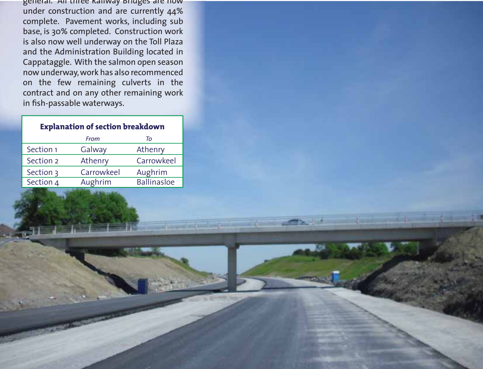
Barnacragh Overbridge which is now open to public use
