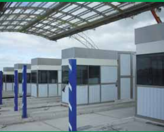
Picture shows the West bound Toll Collection Booths and Optical Barrier Classification poles which will be able to identify all vehicles.
