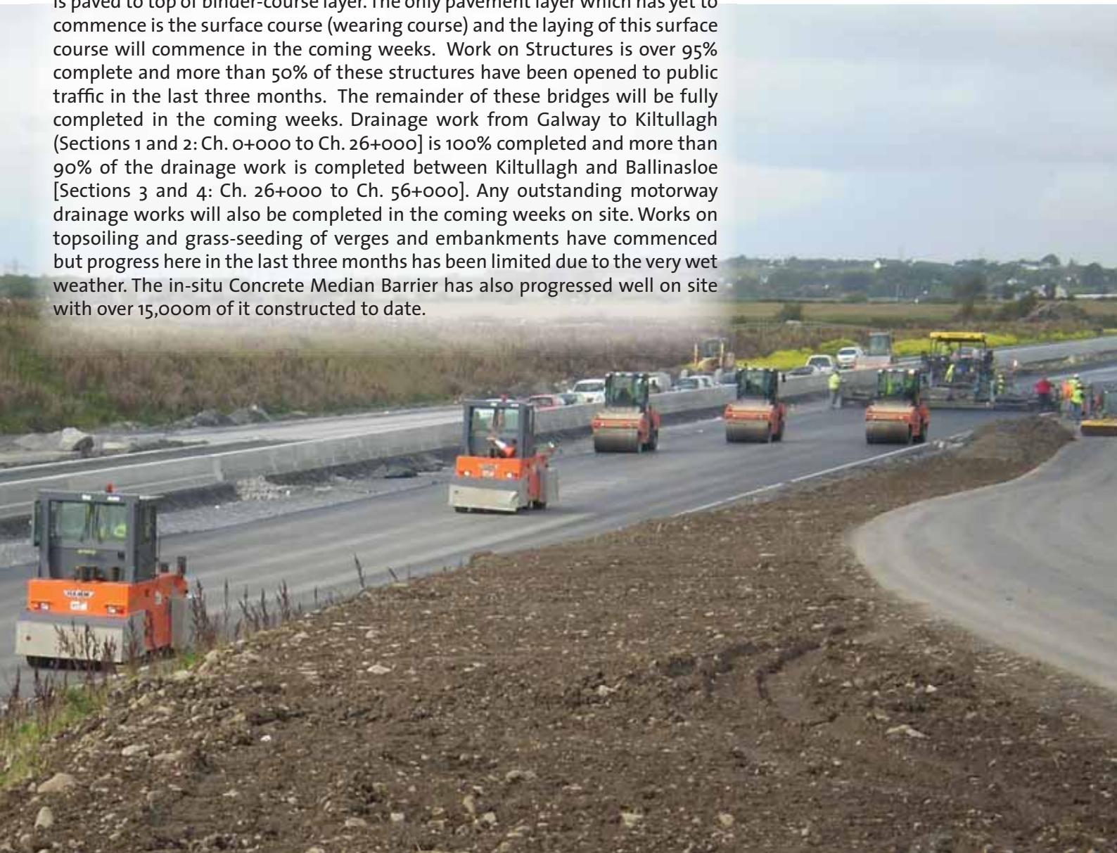
N6/18 Grade Separated Junction – Ch 3+600. Asphalt works taking place after Safety Concrete Barrier Installation.
