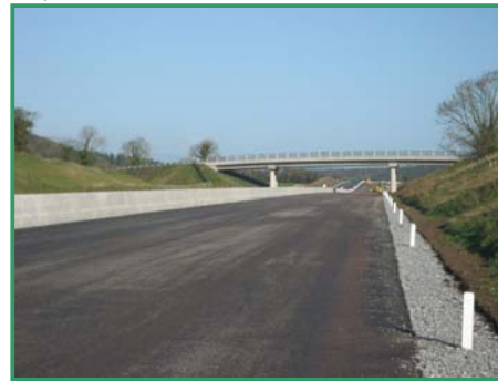
Third Layer Surfacing and Concrete Barrier, Looking North at Mondaniel Road Overbridge
