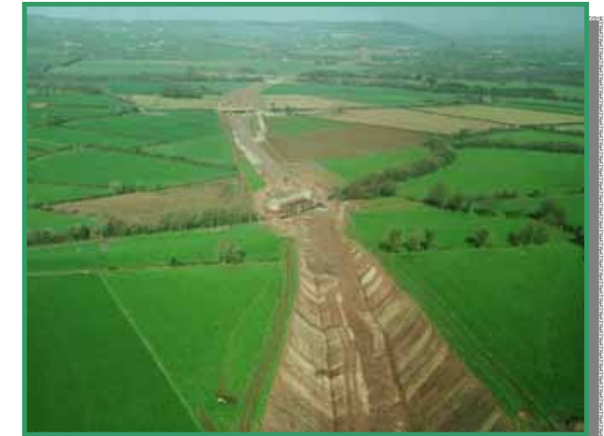
Looking North from the N8 at Rathcormac to the River Bride & Maulane Rd Bridges
