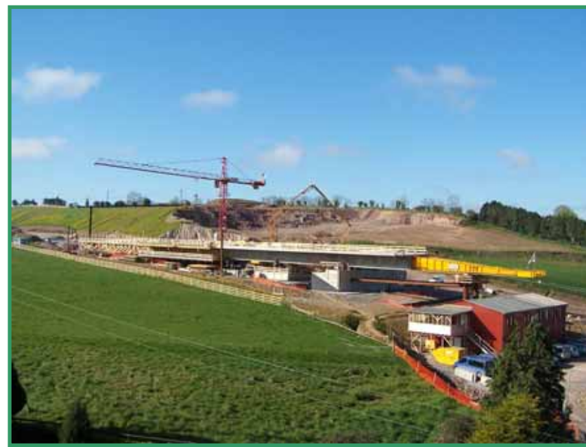
View of viaduct works looking south west, showing deck progress across the valley after the first launches
