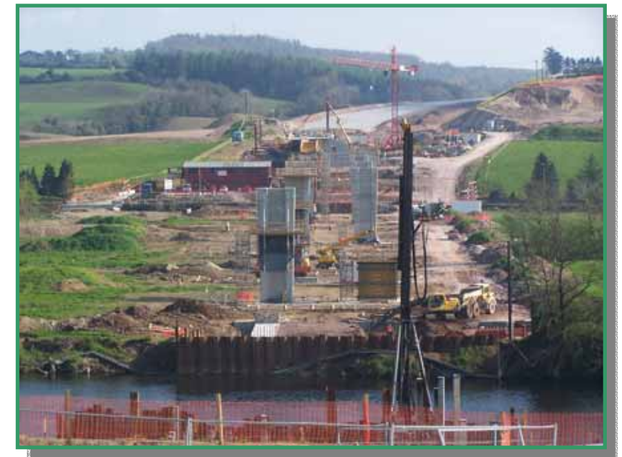
View of the viaduct works looking south from the bank of The Blackwater River
