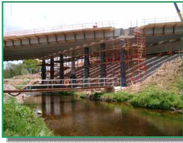
View from the river of the bridge carrying the new N8 over the River Bride
