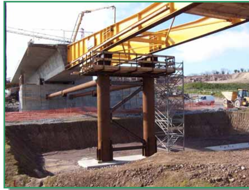
View of the launching nose (in yellow) and the steel temporary support piers.
